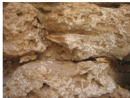
Fig. 3 – Limestone masonry – marine attack.
