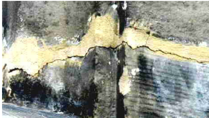
Fig. 4 – “Efflorescence” on natural stone masonry (sediment blocks salts brought to the surface).
