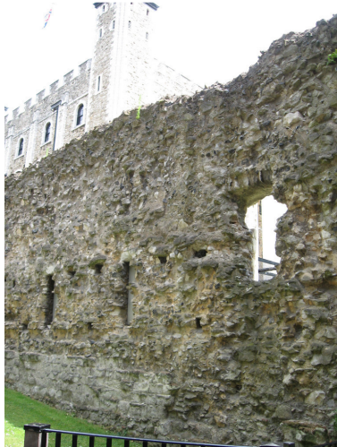
Fig. 2 – Stone masonry subjected to salt attack.
