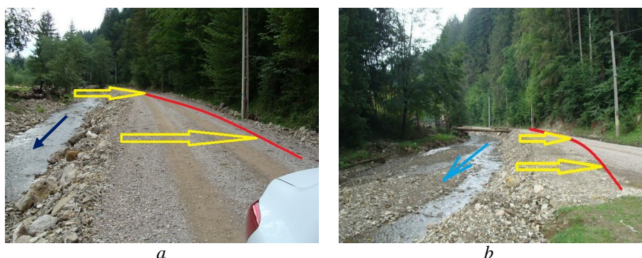
Fig. 5 – Voroneț Stream erosive action on the left bank and DJ 177D road: a – the starting section of the shore defence and road degradation („Camp Cristea” downstream area); b – the ending area of the eroded road section up to the versant (upstream of Brusturos Stream).
