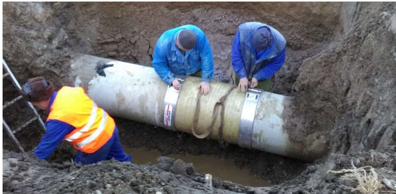
Fig. 4 – The replacement of a 600 mm diameter GRP (PAFSIN) pipe section in Miroslovești locality, Iași county.
