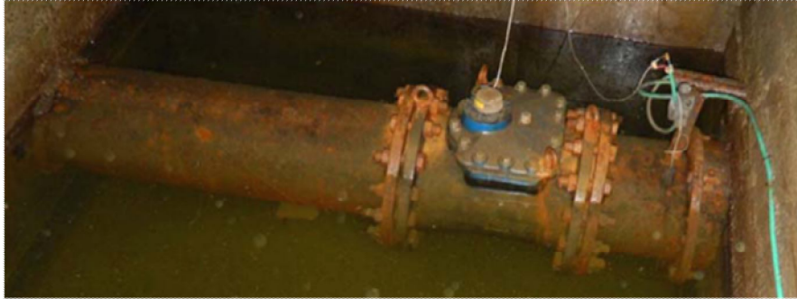
Fig. 3 – Electromagnetic flowmeter fitted to a 400 mm diameter steel pipe inside Cerna pumping station, Iași.
