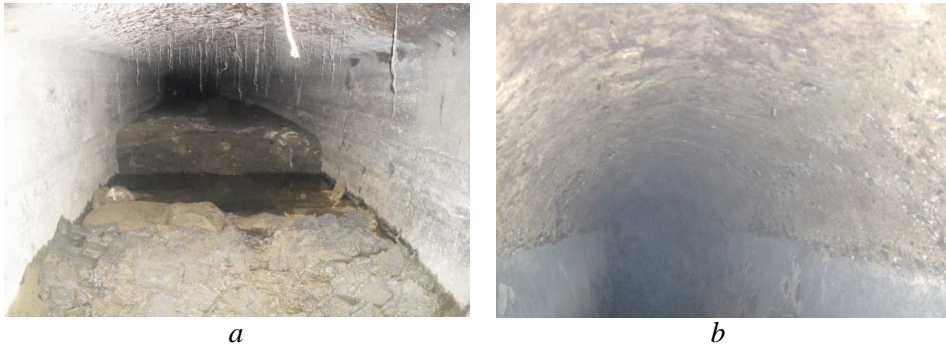
Fig. 1 – Degradation one flow path to the sewage collectors visit: a – clogging invert and cementing material deposits; b – the degradation of concrete soffit plate coverage to a collector type ovoid (Lucaa & Hobjilă, 2005).
